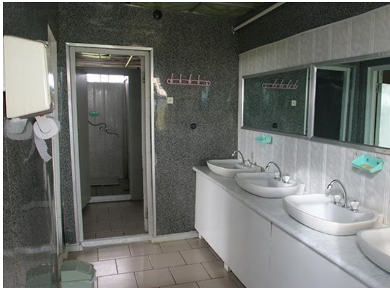
Washing facilities, hot shower & western toilet available
